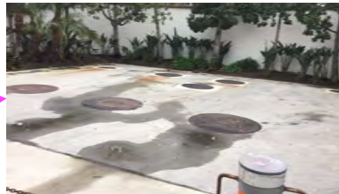
4 drywell hatches below flood level
