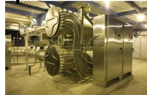
3 Reverse Osmosis with AOP Groundwater Injection
