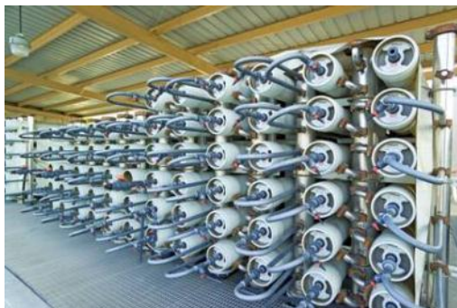
4 Single Pass RO Low-Pressure Boiler Feed
