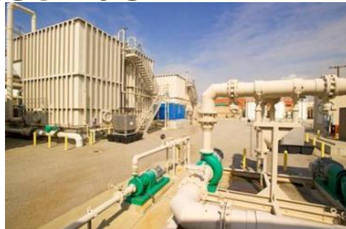
2 Nitrified Water Cooling Towers
