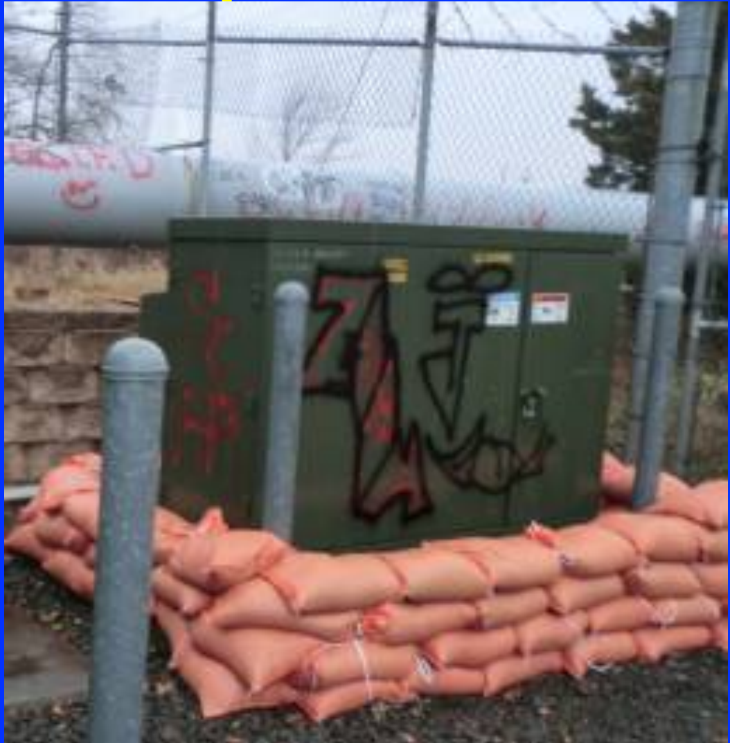
CPS-18 Wrangle Brook Lift Station Transformer (Toms River)
