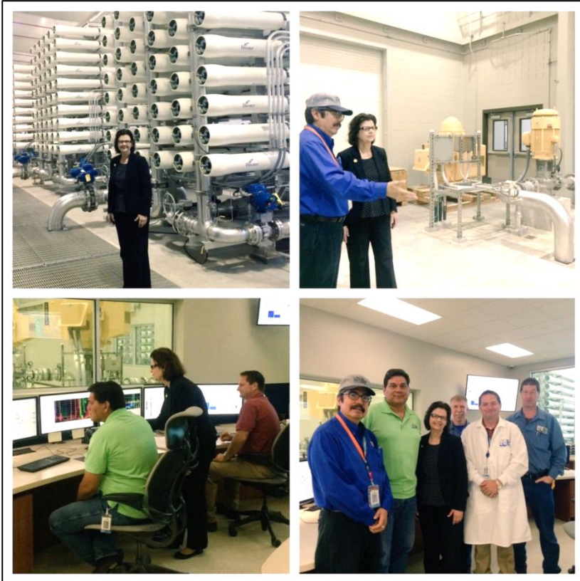
San Antonio Water System (SAWS) H2Oaks Center – Brackish Desal Plant
