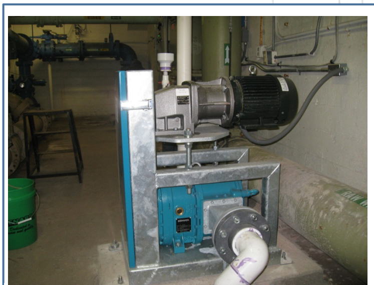
Rotary pumps used for Transfer and Recycle Pumps to minimize damage to living algae
