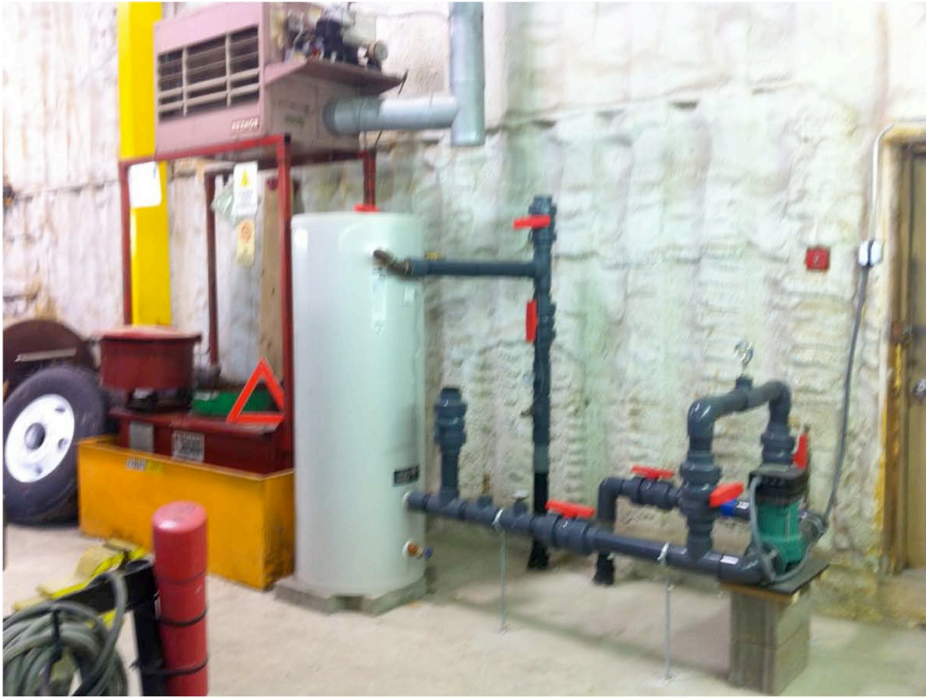
Circulating Pump and Tank in Maintenance Facility
