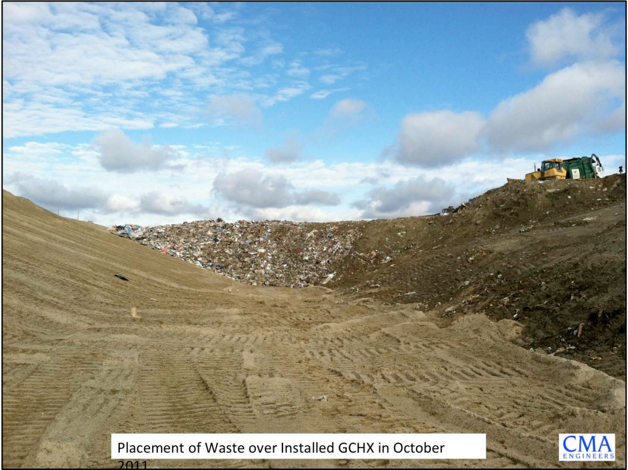
Initial waste placement in October 2011 in Stage IV Phase II-A and over the heat exchanger.
