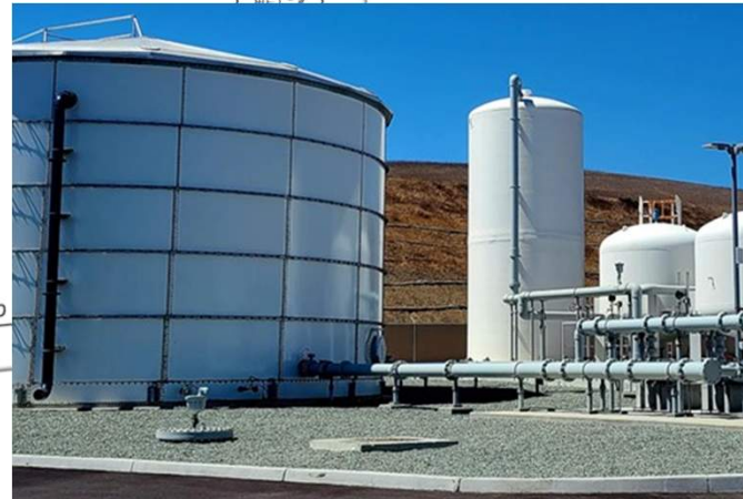
Product Water Tank – 200,000 gallons
