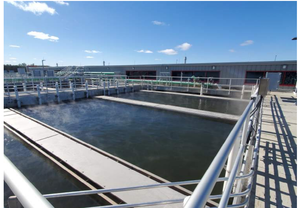
AGS during fill/decant cycle October 31 st
